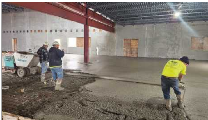
POURING THE CONCRETE floor of the Iron Workers Local 8 Upper Peninsula Training Center in Harvey are Jim Trudeau, Frank Seacott and Robert Lordsen. The Bricklayers and Allied Craftworkers Local 2 members are employed by Gundlach Champion.
