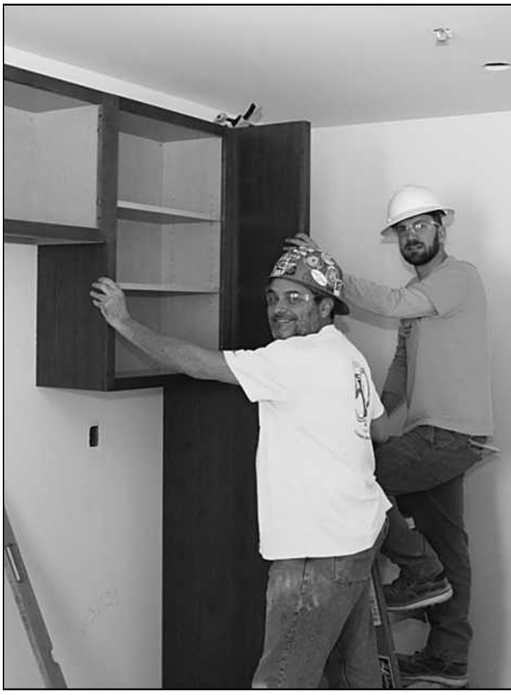
SETTING KITCHEN CABINETS in a 17th floor apartment at the Residences @ 150 Bagley project in Detroit are Michigan Regional Carpenters Council members Kevin Wychuyse (Local 687) and Dominic Sprinkles (Local 1234). They're employed by Landry Carpentry and Millwork.
