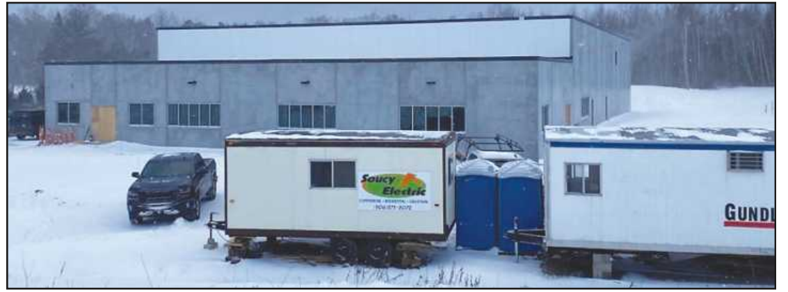
THE 17,136- SQUARE-FOOT U.P. Training Center for Iron Workers Local 8 is enclosed for the winter, and a variety of interior work is ongoing.
